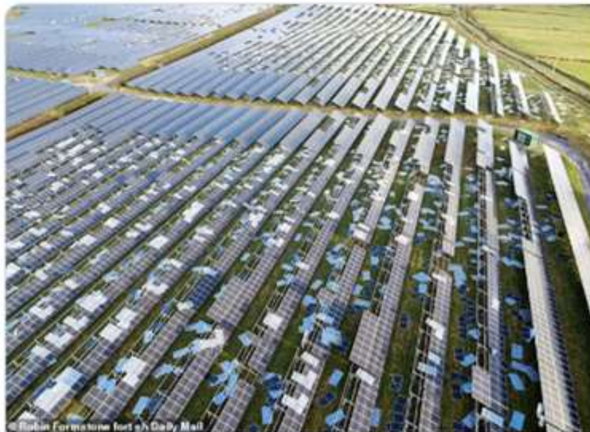
hundreds of solar panels were blown off their mounts and damaged beyond repair
